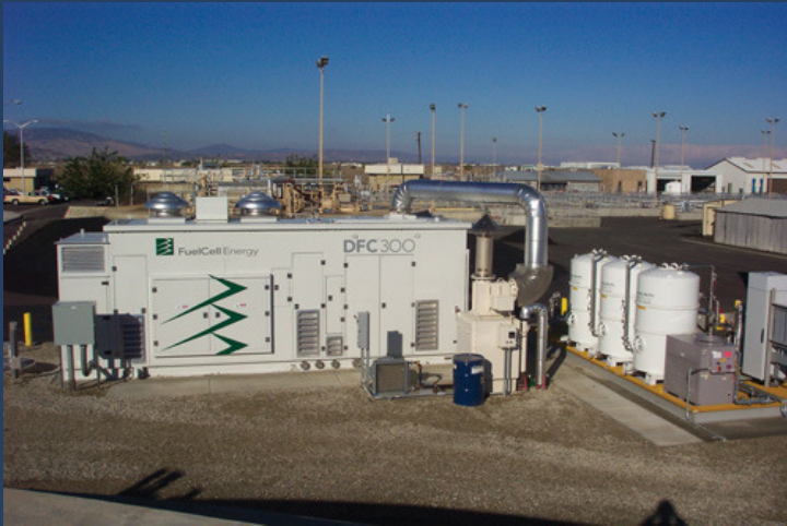
Los Angeles County Sanitation District, Palmdale Water Reclamation Plant
